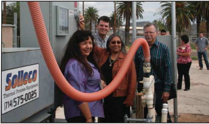
Gila River Indian Community and U.S. EPA Region 9 switch on the new remediation system at an abandoned LUST site.
