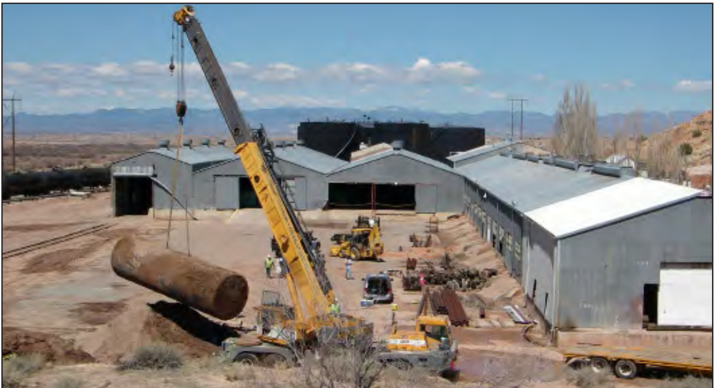
This 10,000-gallon tank was one of three USTs removed during a site assessment at Valero Asphalt, on the Santo Domingo Pueblo, New Mexico.
