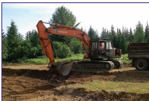
Field screening for PCB levels (top) was used to guide the site excavation (bottom).
